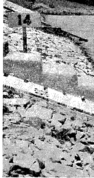
A section of the earthen dam. Below: water channel being lined with cement concrete
