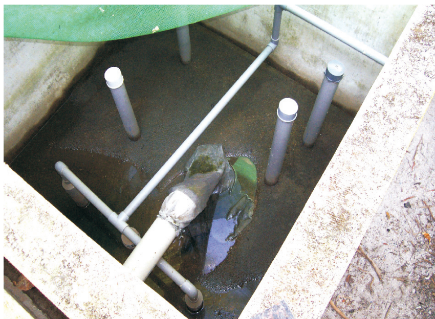
This system is innovative when compared to any other rainwater system seen in coastal parts of India.
