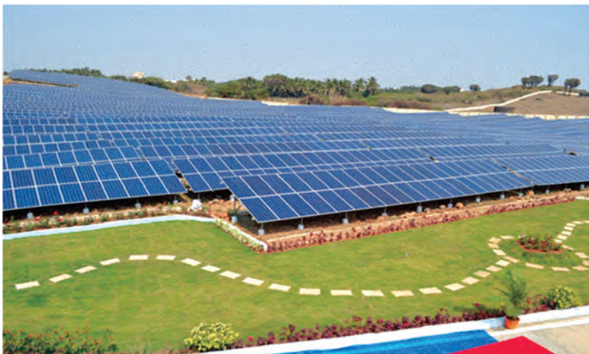
Solar PV Installation, Diu Smart City
