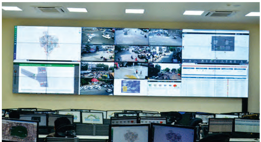
Integrated Command and Control Center at Vadodra
