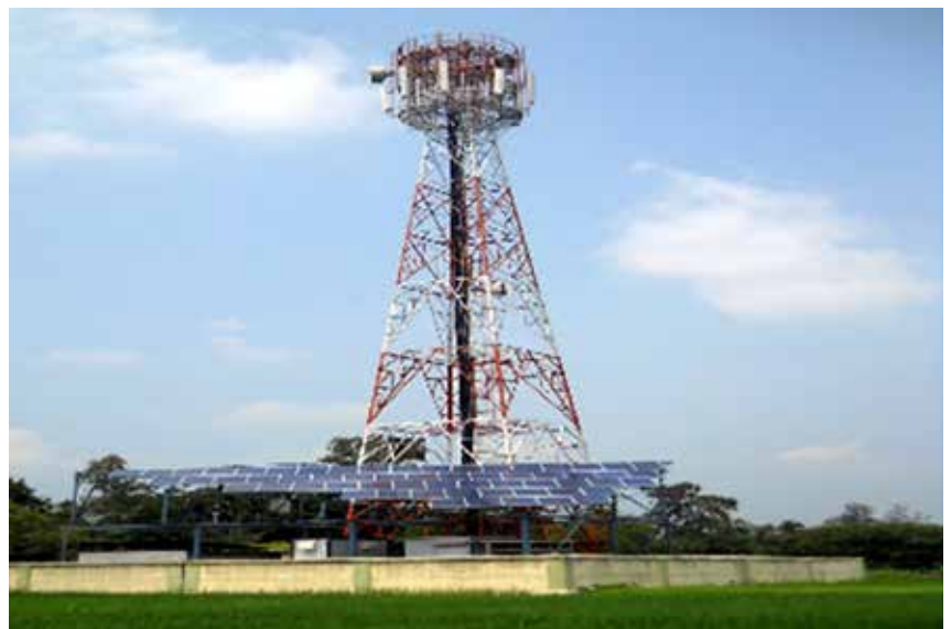
Hybrid power supply to telecom towers
